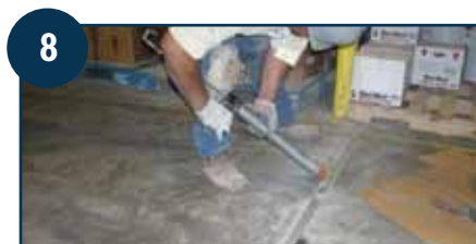
8 Additional grinding, filling and finishing may be necessary to complete the repair.
