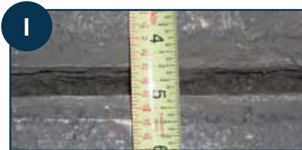
1 Survey slab, measure and record deflection (optional), determine location for installation and repairs.
